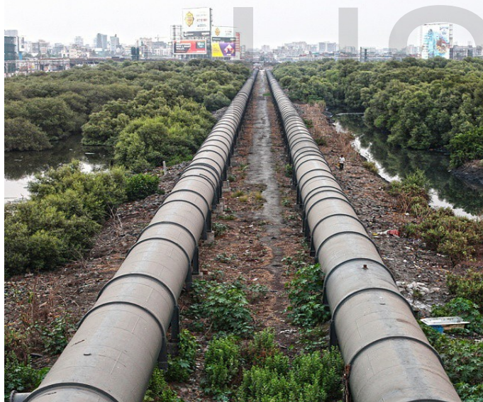
Fig- Mahim-Bandra Water Pipeline
